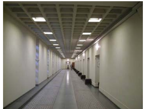
20 W tungsten halogen lamps above the doors replaced by 2 x 3 W LEDs
