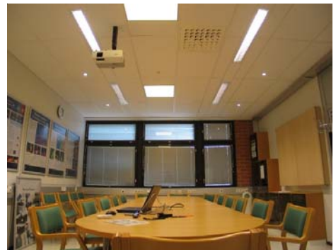
Lighting by a combination of LED and fluorescent lamps in the meeting room
