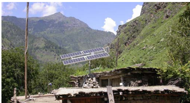
Solar electricity for lighting in remote Nepali village.
